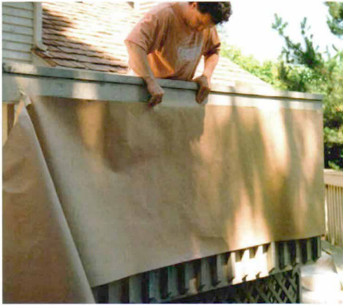
Keeping overspray under control. The author covers the deck with tarps, wraps the first floor of the house with plastic sheeting and masks the outside of the railing. After coating the inside of the railing, he'll remove the paper and spray the outside.
